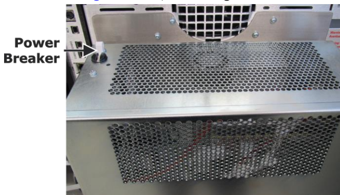
Figure 3-95 Control Box Power Breaker
