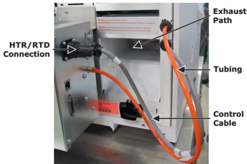
Figure 3-107 Control Cable and Tubing Installed to Control Box
