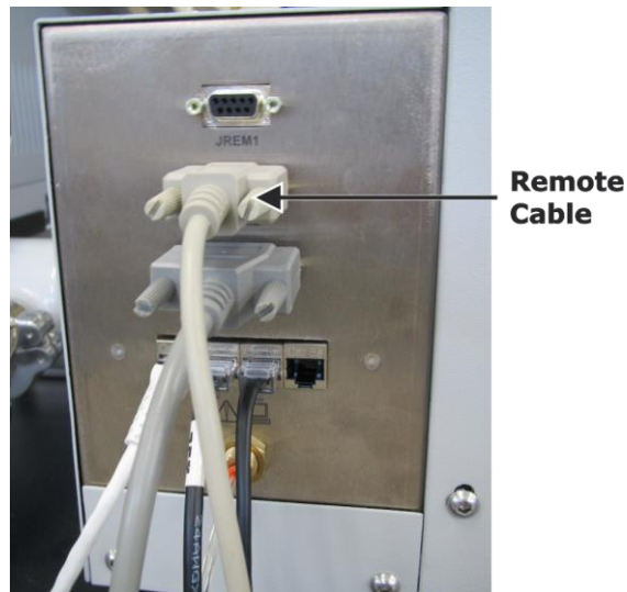
Figure 3-123 Remote Cable Connected
